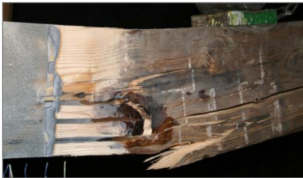
Fig. 25. Failure mode of beam F2
