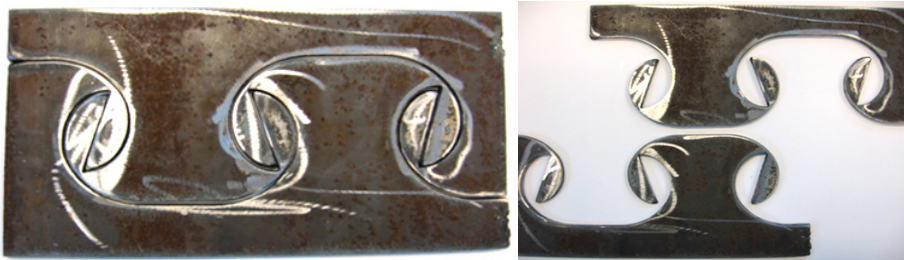
Fig. 3. Steel plate after gas cutting-remaining steel parts to be removed by hand cutting
