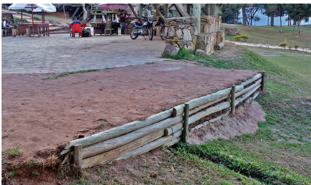
Fig. 10. A contemporary example of a terrace enlargement with a wooden wall and backfill (photo by J. Kościuk)
