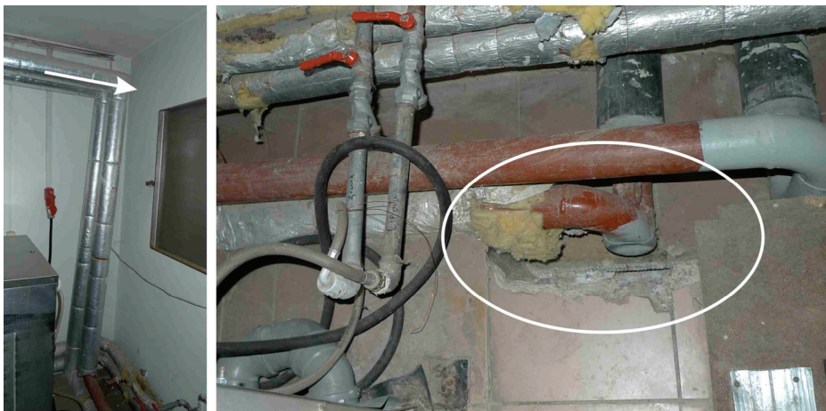
Fig. 17. NH laundry room. Visibly bent pipes and incuts made to protect the piping from damage
