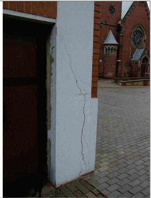
Fig. 13. Cracked wall near South-West corner of the Nursing Home
