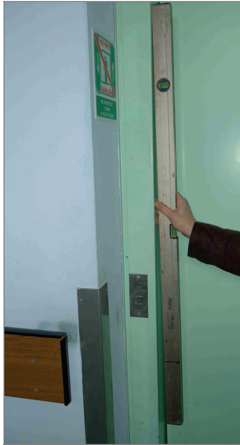
Fig. 14. Vertical tilt of lift shaft
