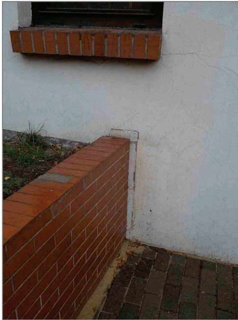
Fig. 12. Displacement of the building illustrated by original location of retaining wall
