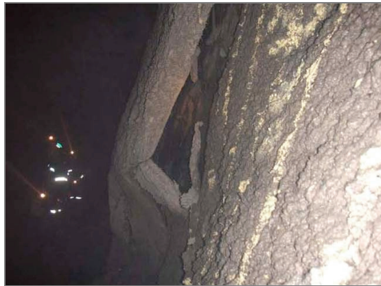
Fig. 10. Support is too stiff to the intended ground deformation
