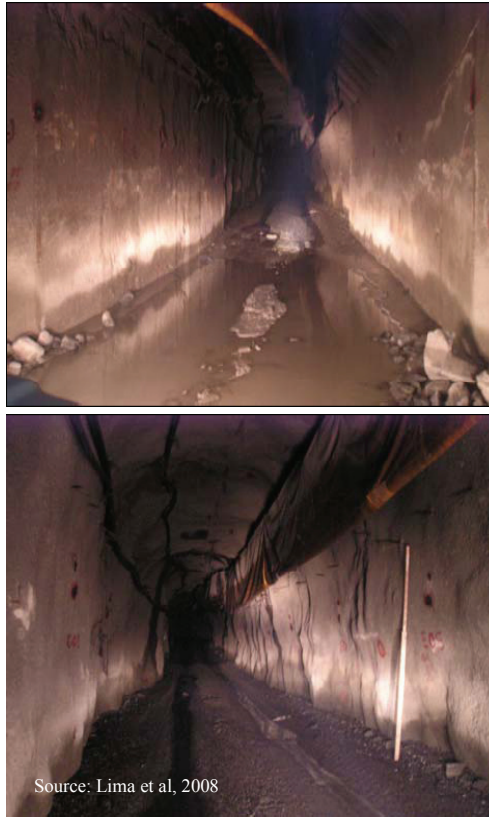
Fig. 12. Example of steel sets and concrete support (top) vs. cable bolting and shotcrete (bottom)
