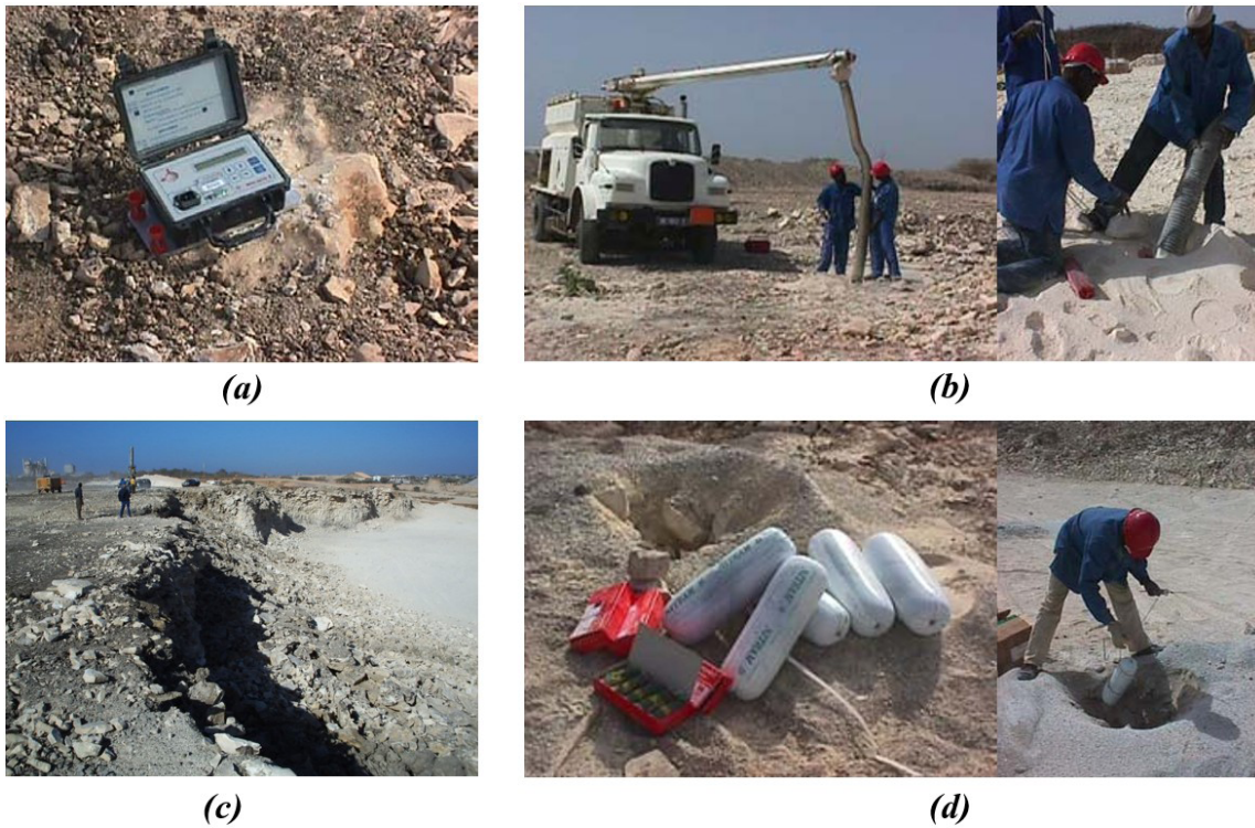
Figure 2: (a) Vibration monitoring sensor; (b) ANFO truck loader; (c) Blast area inspection; (d) Bottom charge with cartridges and electric detonators.
