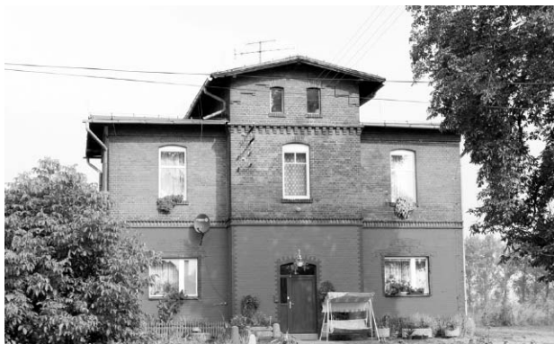
Fig. 2. Lubrza station. The building has been transformed into living quarters. Windows on the ground floor have been rebuilt and all the frames have been ineptly exchanged. The ground floor elevation has been painted (photo: M. Konopka, 2009)
