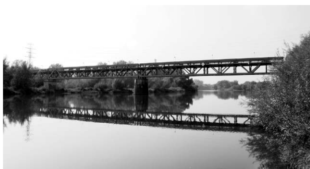
Fig. 4. The railway bridge over the Oder between Krapkowice and Otmęt. The western span fell down during the July 1997 flood. It was repaired but the traffic has not been restored (photo: M. Konopka, 2009)
