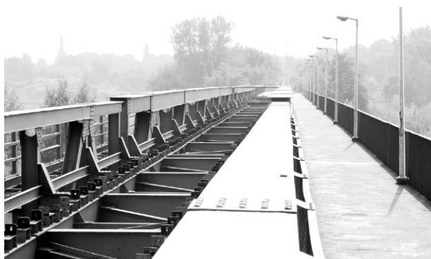
Fig. 5. The pedestrian footbridge on the railway bridge over the Oder between Krapkowice and Otmęt. The track was removed after the July 1997 flood. A pedestrian footbridge has been in operation here since the 1930s. At present the reconstruction of the bridge into a road one is under consideration (photo: M. Konopka, 2009)
