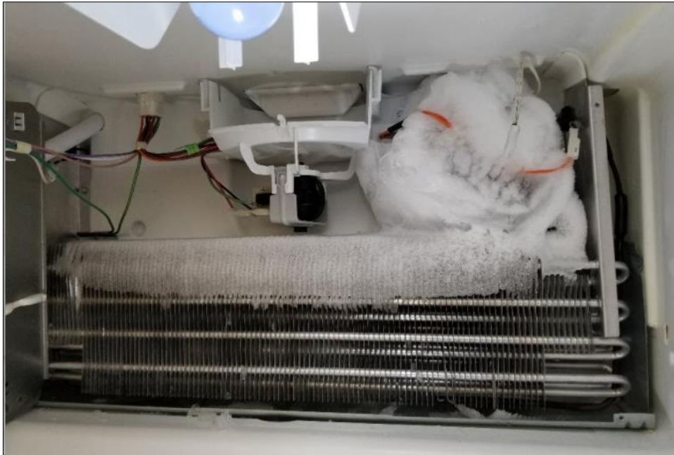
Fig. 1. View on frost accumulated on the evaporator of the refrigerator
