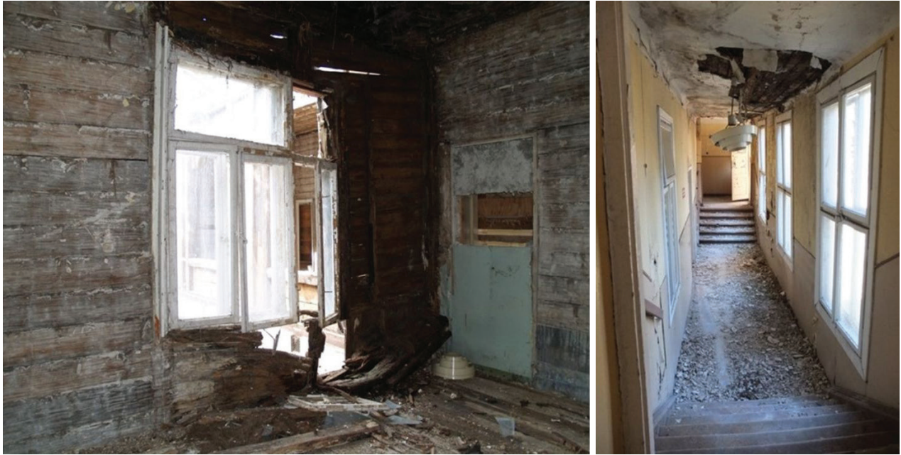
Fig. 5. Biologically corroded wooden walls and ceilings of the Abram Gurewicz Health Resort – condition in 2015 (source: archive of the Grupa 5 Architekci)
