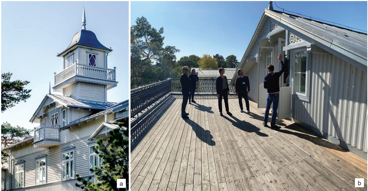
Fig. 8. Elements of the Abram Gurewicz Health Resort recreated on the basis of archival photos: a turret (a) and a sun terrace (b) in the northern wing of the building (photo by A. Grzesik, K. Mycielski, archive Grupa 5 Architekci)
