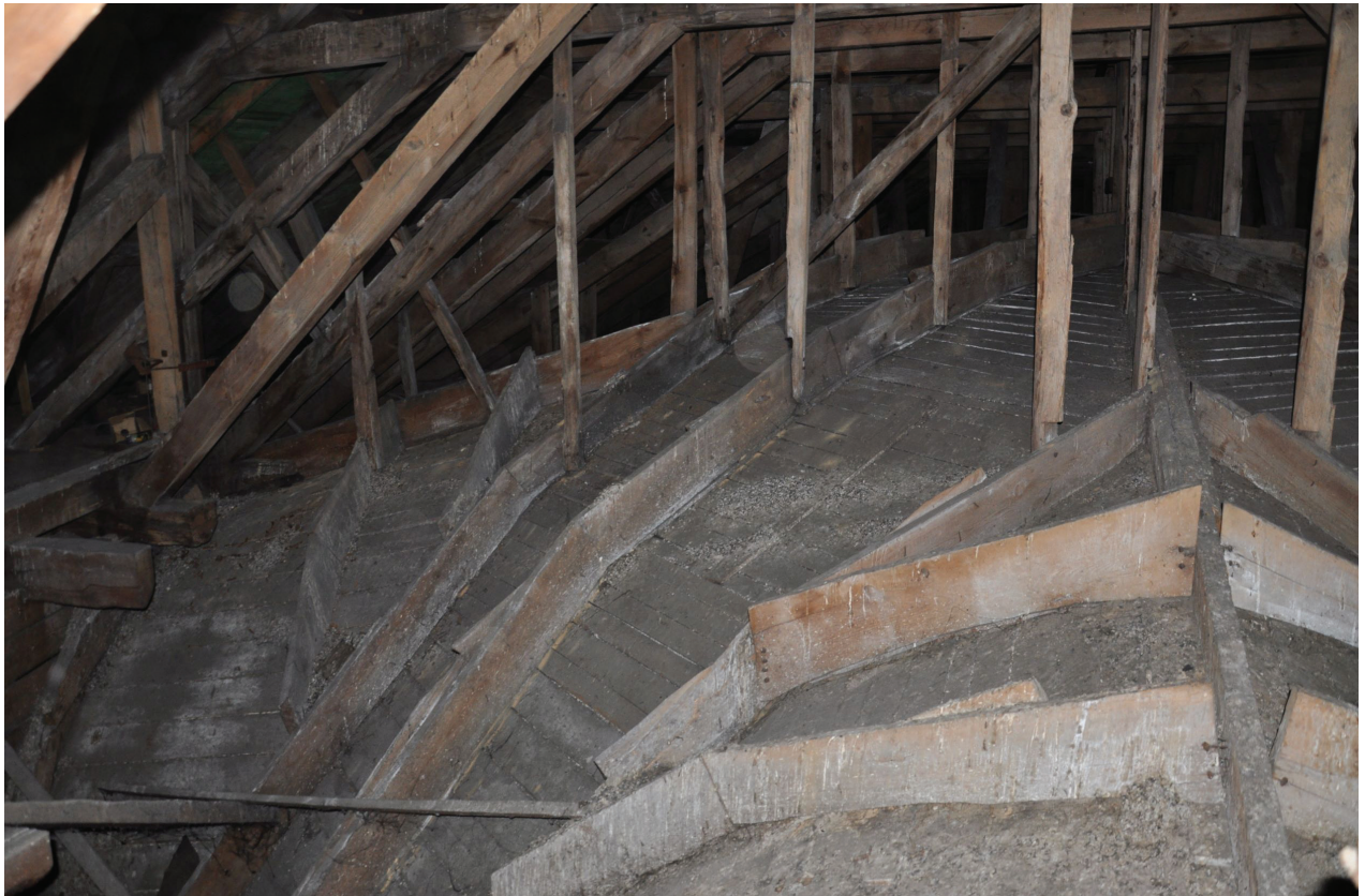
Fig. 2. Leszno, Church of the Holy Cross, roof structure, curved plank roof, curved planks suspended from the structural elements of the roof structure above (photo by U. Schaaf, M. Prarat)
