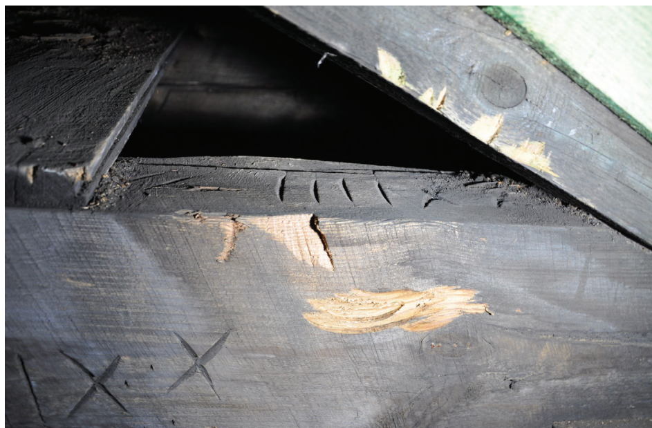
Fig. 14. Leszno, Church of the Holy Cross, roof structure, carpentry assembly marks on both sides of the timber framing (photo by U. Schaaf, M. Prarat)
