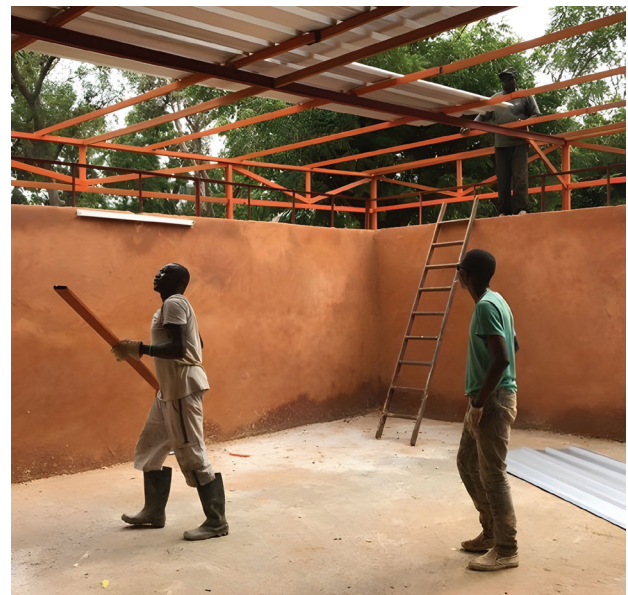
Fig. 7. Primary School, the Quartier Dixième, Thiès, Senegal. Roofing structure (source: image courtesy Let's build my school – humanitarian organization)
