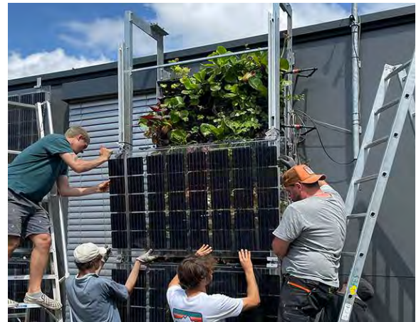
Figure 10: Façade test stand. Installation of centre vertical PV module in front of Kramer greening system / variant 1 (06/2022).
