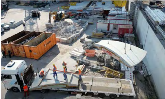
Figure 6: Image: Removal transportation of formwork elements from the main station Stuttgart building site ©DB AG
