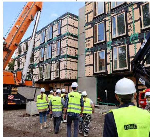
Figure 1: The technology demonstrator building during construction, prior to external facade finish application; photo courtesy of DMDmodular p.s.a.
