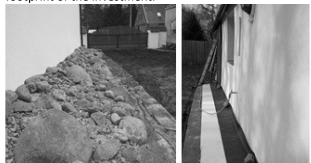
Figure 8, 9: Insulation of the foundation following the schemes (after/during work); Condition approx. 2020, source: author
