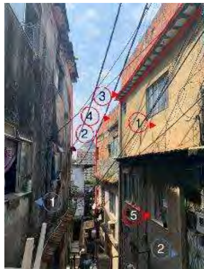
Figure 2: Case-Study 1 – Alley Building. Typical narrow street in Community Morro Azul, RJ. Photo: P. Paixao.
