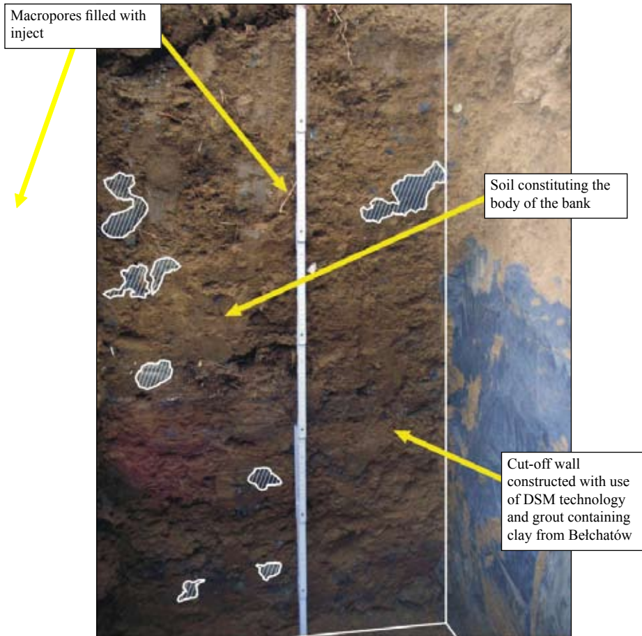
Photo 25. Exposed wall of the soil in the body of the bank. Places, where inject filled the macropores of soil outside of the zone of the cut-off wall are marked
