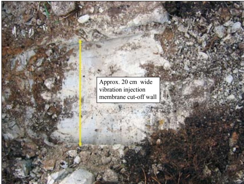
Photo 20. Crown of the embankment: exposed membrane cut-off wall constructed with use of vibration injection technology with the inject made from clay from Bełchatów
