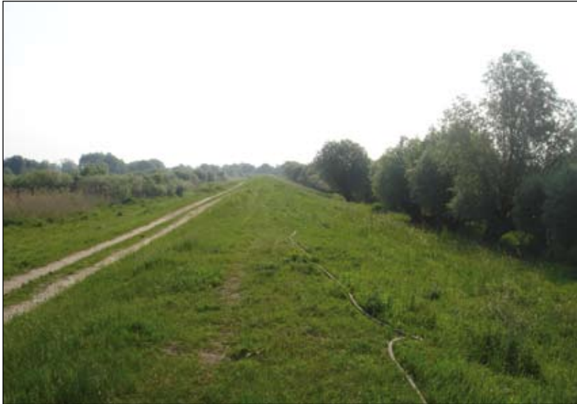
Photo 13. View of the section of embankment where the section of cut-off wall was to be constructed
