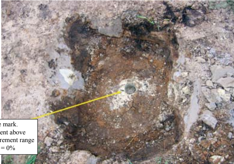
Photo 24. Mark of the CBRd plunge on the surface of the cut-off wall constructed with use of vibration injection technology from inject based on clay Belchatów
