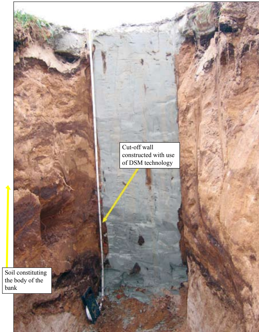
Photo 21. Open pit No. 4 – cross-section through the cut-off wall constructed with use of DSM technology grout based on clay Bełchatów
