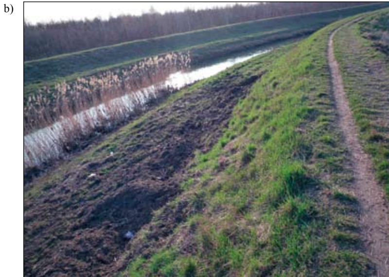
Photo 1 (a, b) Embankments of the river Śleza devastated by boars
