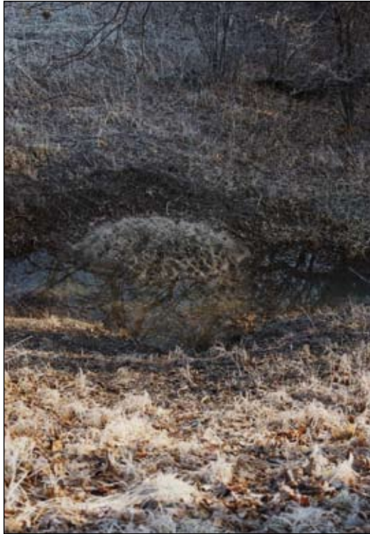
Photo 4. Zone of non-cohesive soil loosened by filtrating waters (piping)
