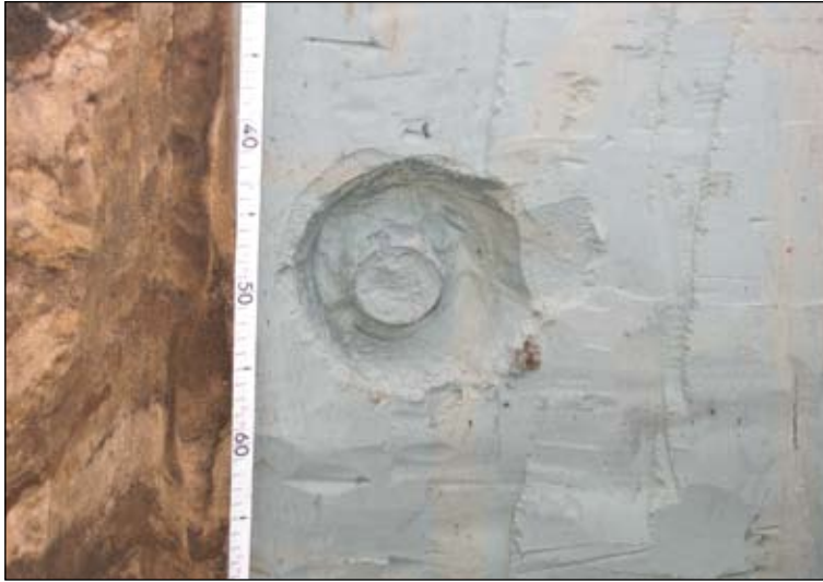
Photo 23. Open pit No. 4 – exposed cross-section through the bank on the contact point with the cut-off wall constructed with use of vibration injection technology from grout based on clay Belchatów
