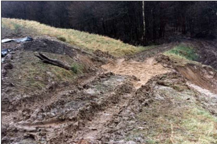
Photo 11. Crown of the flood banks driven over by cars – lack of service road
