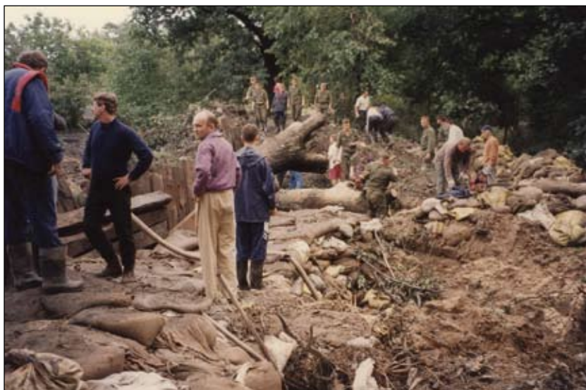
Photo 7. Gap in the flood bank on Odra created as a result of a tree falling down
