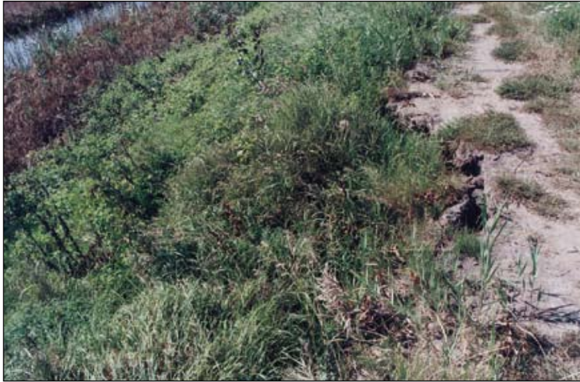
Photo 2. Subsidence of the crown of the bank
