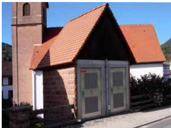
Ryc. 2.20. Trafostacja zlokalizowana w pobliżu kościoła we wsi Nothweiler, 2004 Fig. 2.20. Power transformer station located in the neighbourhood of the church in Nothweiler village, 2004
