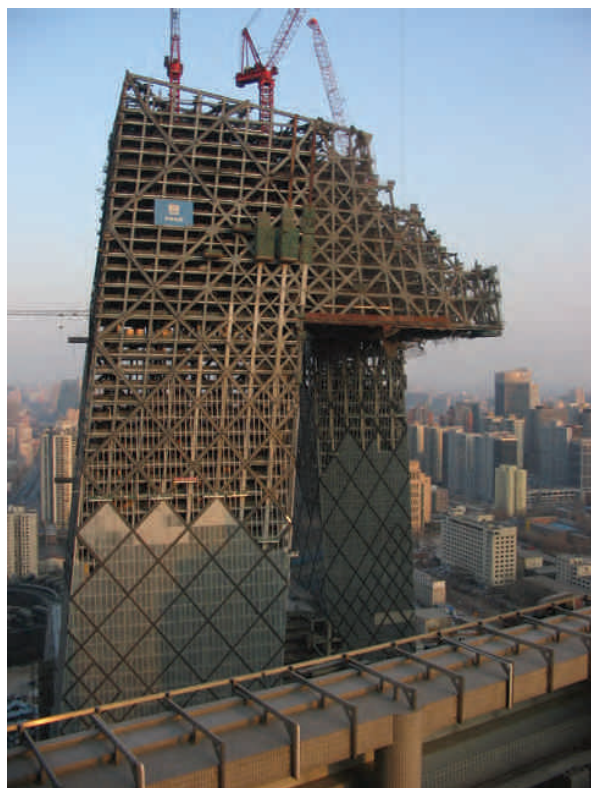
Fig. 7. Seat of CCTV in Beijing under construction (February 2008) designed by OMA. Futuristic structure is one of the 'icons' of modernized capital city of China (photo: J. Krajewska)
