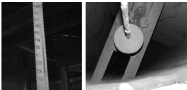
Fig. 6. Installed float near the column
