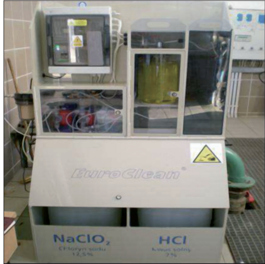
Photo 2. Chlorine dioxide generator installed at the water treatment station in one of Wrocław's hospitals
