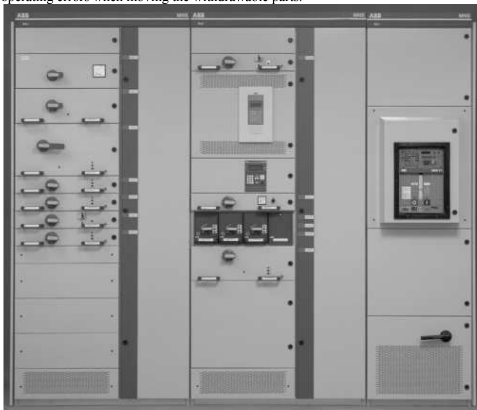
Fig. 9.4. MNS switchboard in industrial plant
