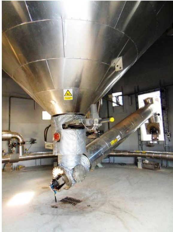
Figure 7-17 Conical outlet of a Dranco digester with an extraction screw
