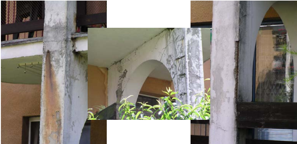
Fig. 1. Example of loggia structure damage
