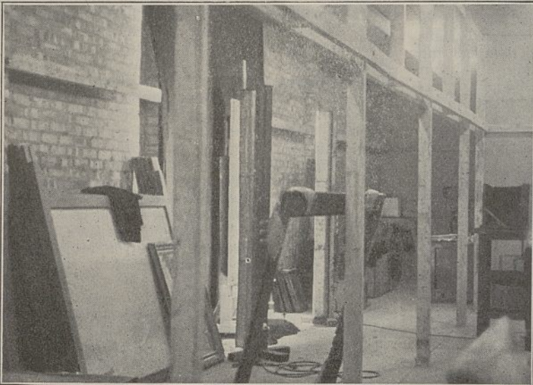
Fig. 3. PART OF A STORAGE CHAMBER BEFORE OCCUPATION, SHOWING STACK OF SCREENS (LEFT), READY TO BE FIXED BETWEEN THE UPRIGHTS IN CENTRE.
