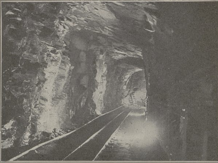
Fig. 1. THE MAIN UNDERGROUND APPROACH LEVEL. THIS WAS ORIGINALLY OF CROSS-SECTION 6 FT. \times 6 FT. AND WAS ENLARGED TO 13 FT. 6 IN. HIGH AND 10 FT. WIDE.
