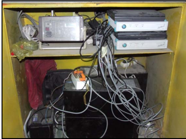
Fig. 1. The interior of the equipment cabinet at an underground test position („Spider 8” measuring amplifiers, portable computers and UPS power supplies shown in the picture)
