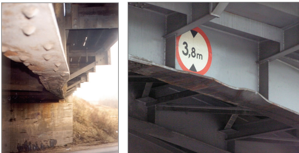
Fig. 2. Deformations of bridge plate girders
