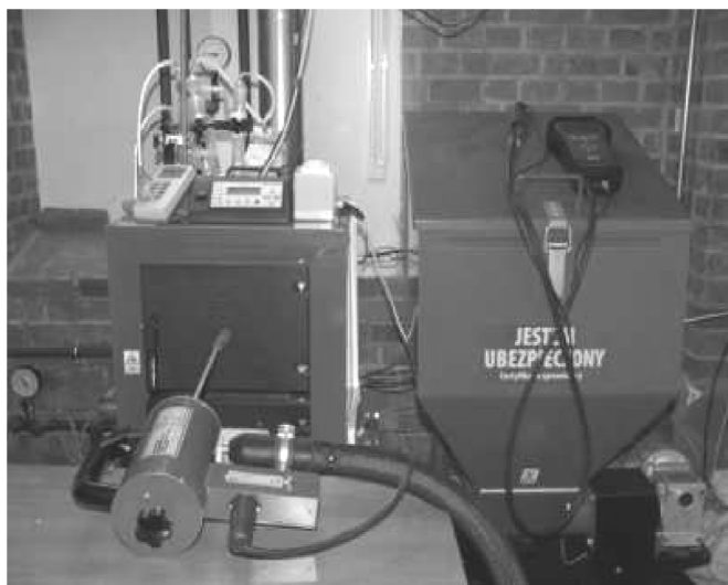
Fig. 1. The water boiler during taking measurements
