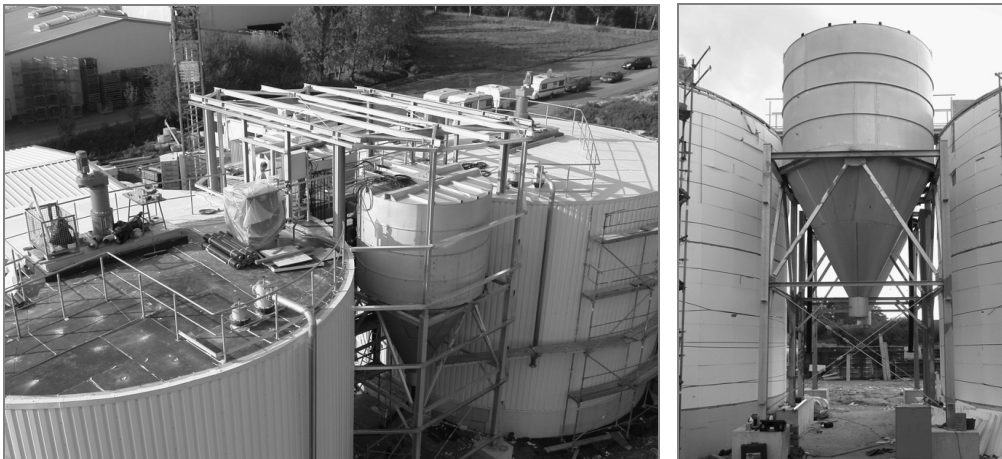
Fig. 6. View of digester and SER reactor at Gemüse Meyer treatment works
