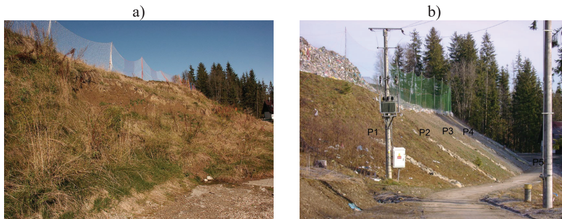
Figure 2: Landfill retaining embankment: a) damaged, 2004, and b) after repairs with counterforts P1–P5, 2005.
