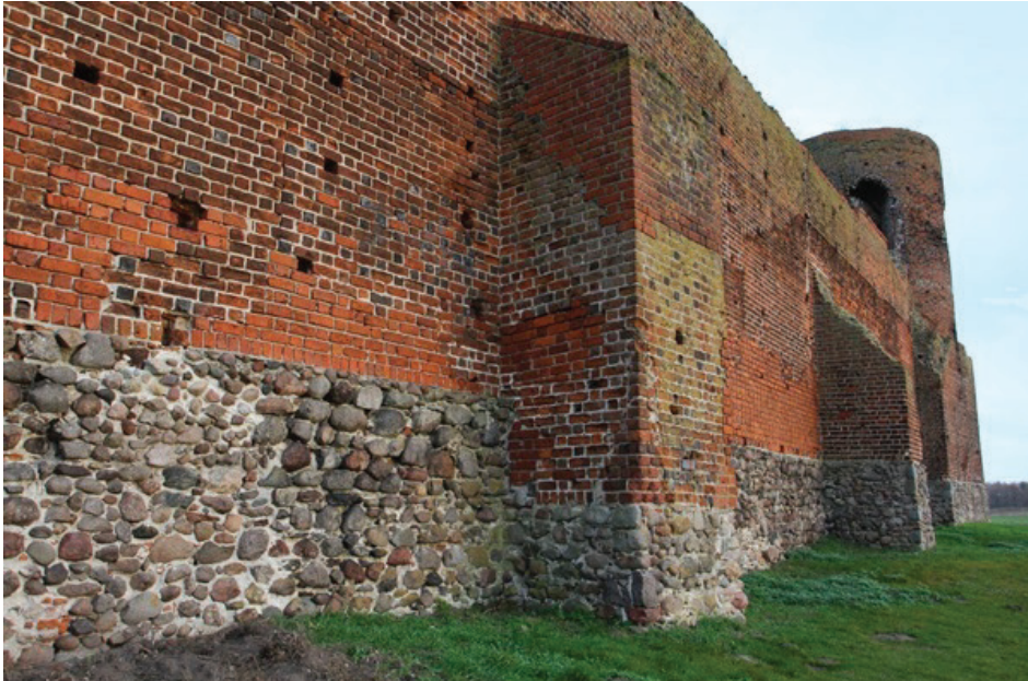
Fig. 10. Castle in Koło. A fragment of the outer façade of the west wall – visible extensive restorations of brick and stone faces as well as microbiological layers (photo by A. Gralińska-Grubecka, 2020)
